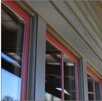
Window sash & frame appear as real wood
