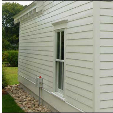
Eaves with no gutters & drip zone
