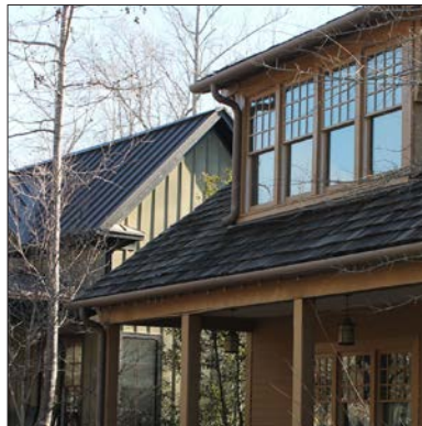
Half-round gutters on non-return eaves
