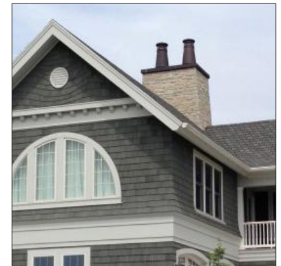
Simple metal flues painted black
