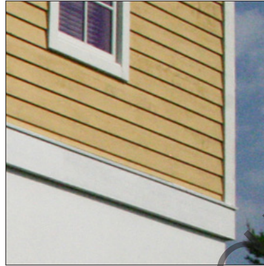
Face of studs aligns with base
